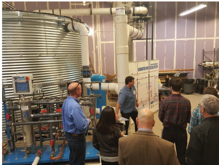
Group tour of rainwater harvesting system. Photo credit: Mitchell Cookas
